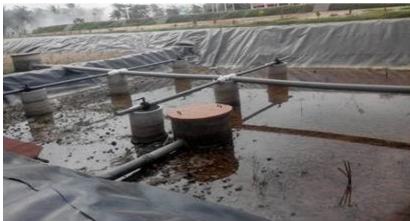
Figure 5. 11 Constructed wetland no. 8 (vertical flow) at Khulna FSTP
