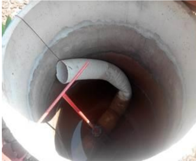
Figure 5. 9 Receiving tank at Khulna FSTP
