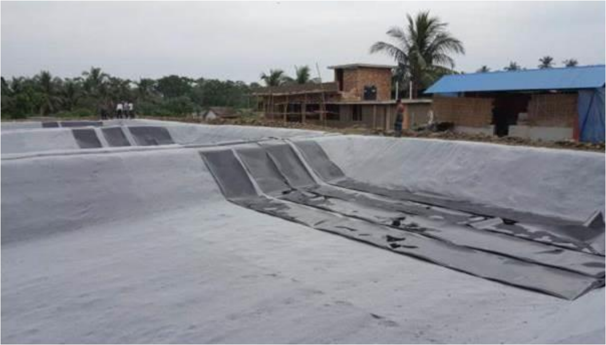
Figure 5. 2 Use of Geotextiles and High Density Polyethylene (HDPE) sheet over the basins of FSTP
