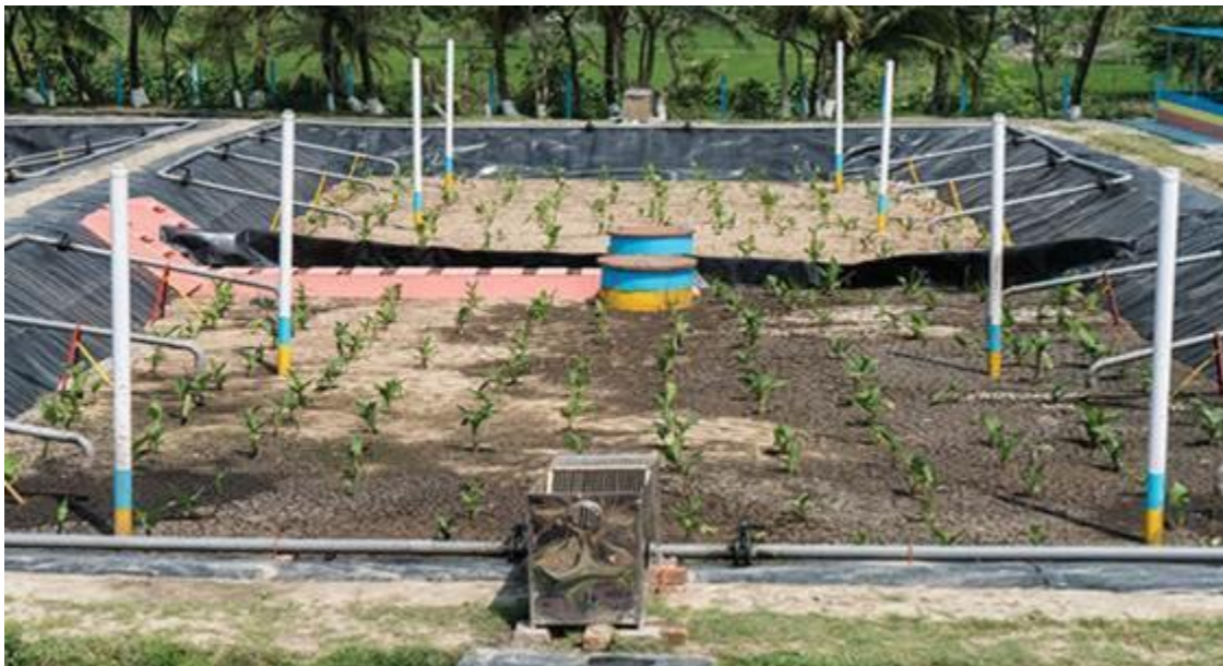
Figure 5. 3 Startup phase at Khulna FSTP
