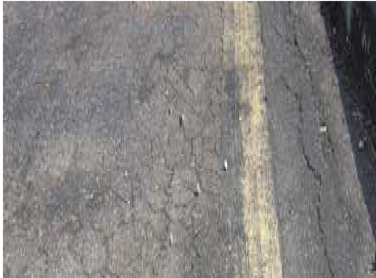
Figure 2.9: Photograph of rutting
