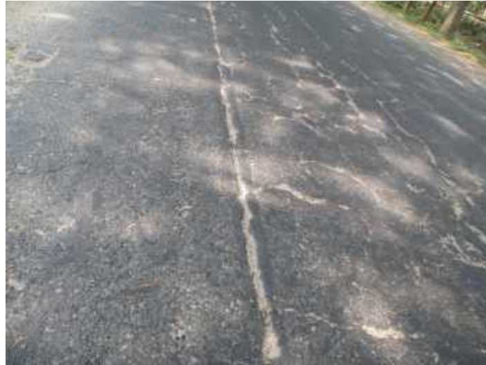
Figure 2.5: Photograph of longitudinal cracks
