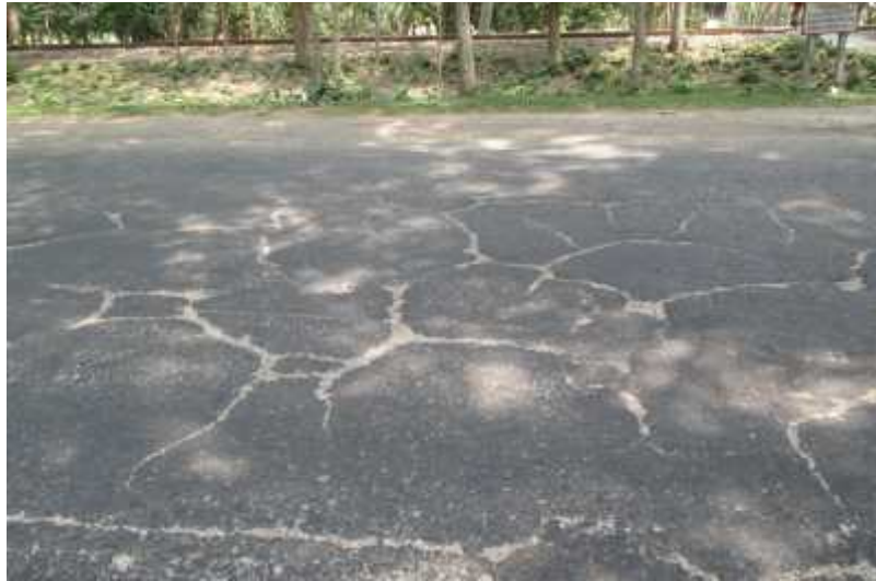
Figure 2.4: Photograph of block cracks
