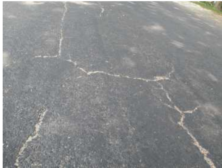
Figure 2.6: Photograph of transverse cracks
