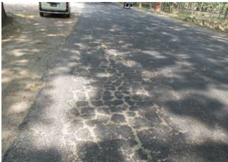
Figure 2.3: Photograph of alligator cracks
