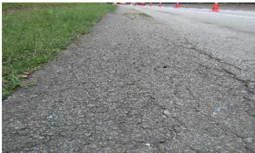
Figure 2.8: Photograph of Edge Cracks
