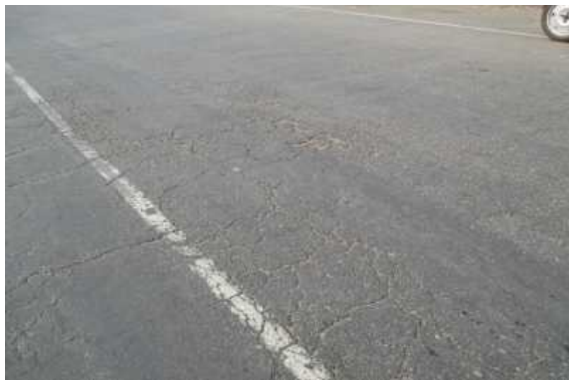
Figure 2.7: Photograph of crescent shaped cracks
