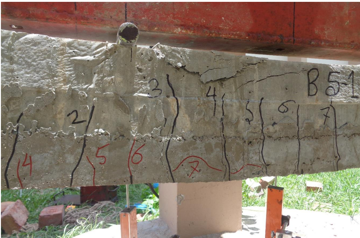
Figure 5.20: Failure mode of beam strengthened with steel angles (B5-1)
