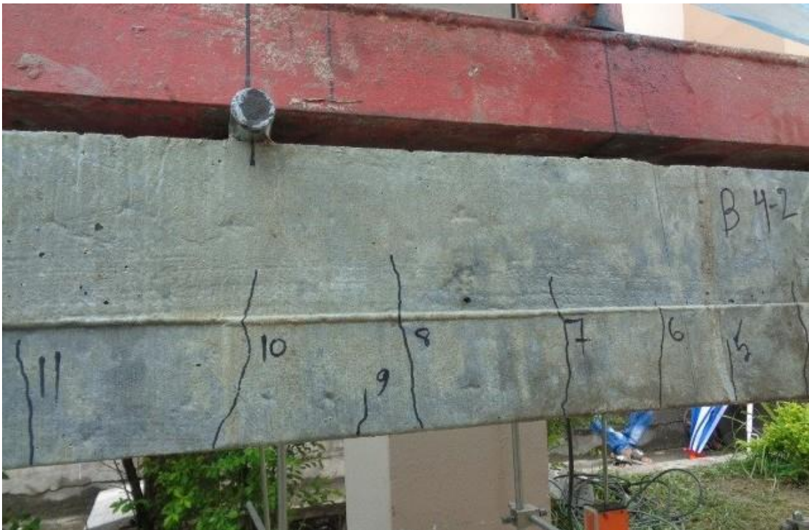
Figure A-12: Crack pattern for preloading (B4-2)
