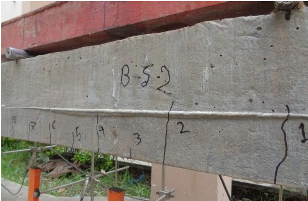
Figure A-16: Crack pattern for preloading (B5-2)
