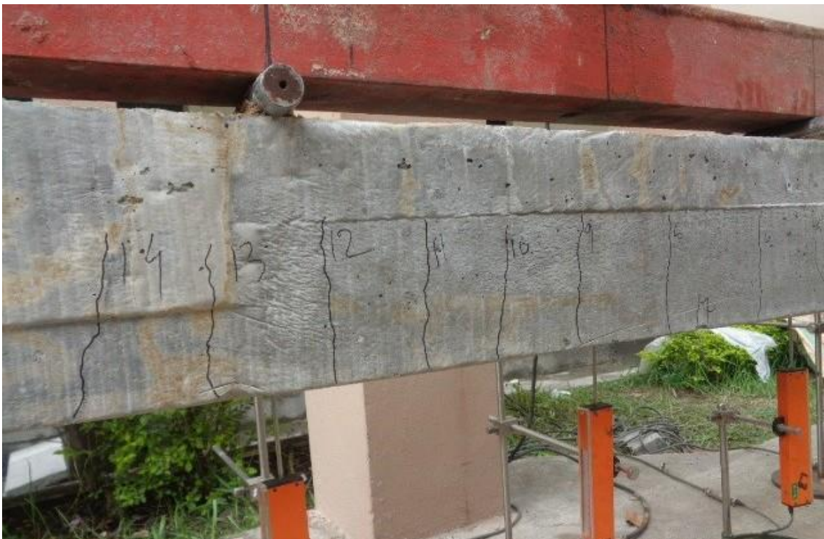
Figure A-10: Crack pattern for preloading (B4-1)
