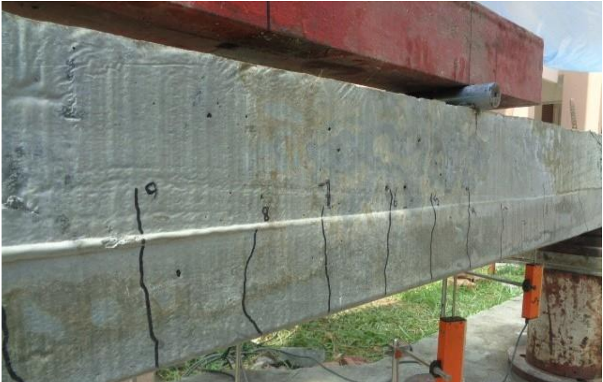
Figure A-2: Crack pattern for preloading (B2-1)
