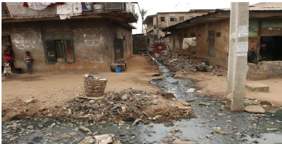
Figure 2.7: Environmental Impacts on Drain Blockage by Shoe/sandal Waste
