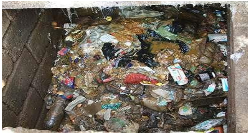
Figure 2.3: Photographic View of Drain Blockage caused by Waste Shoe/sandals
