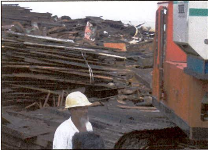
Picture -7 : Stacking of Metal Plates according to size and Quality
