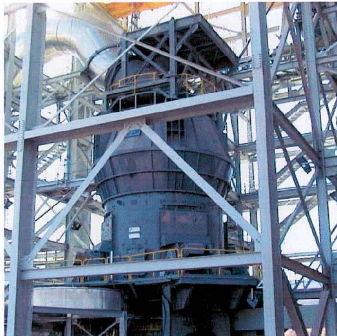
Fig 3.2 Vertical Roller Mill
