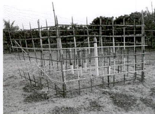
Figure 4.15 Landfill gas monitoring pipe
