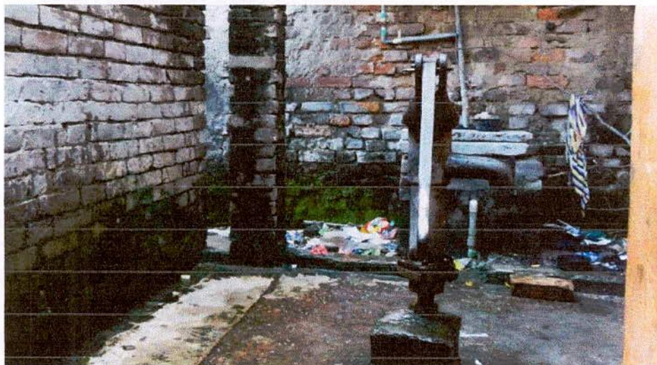
Figure 4.5: Disposal of solid wastes nearby drain and tube-well premises at Shekh Bari Modina Masjid, Motlober Mor.
