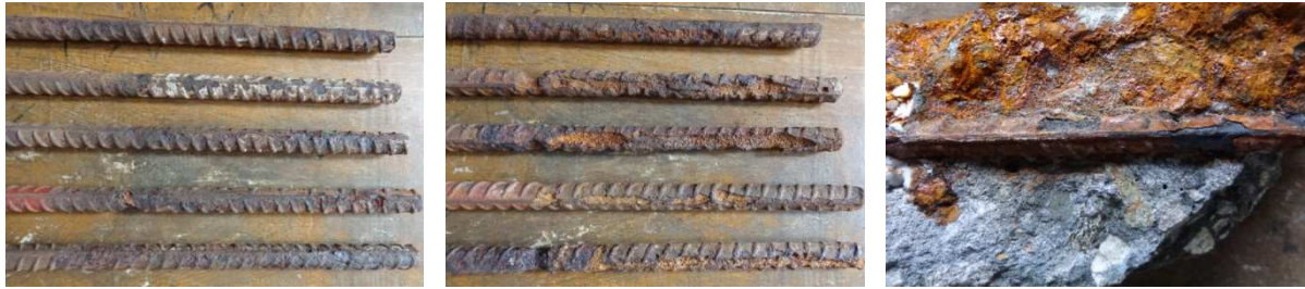
Figure 4.27: Corroded reinforcing steel
