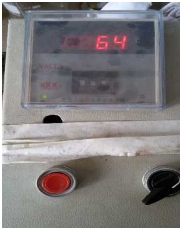
Figure 4.4: Photographic view of Temperature controller
